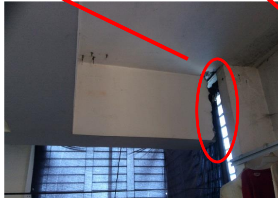
Exposed reinforcement at end of cantilever beam supporting 7 th Floor (Roof) slab
