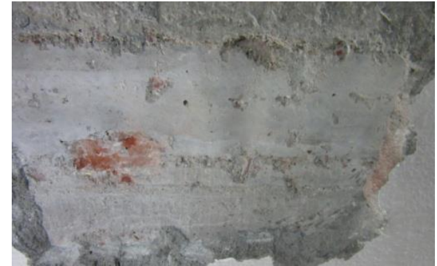
Tested Ground Floor Column – Brick Chips
