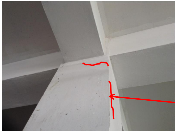
Cracking on column at second floor
