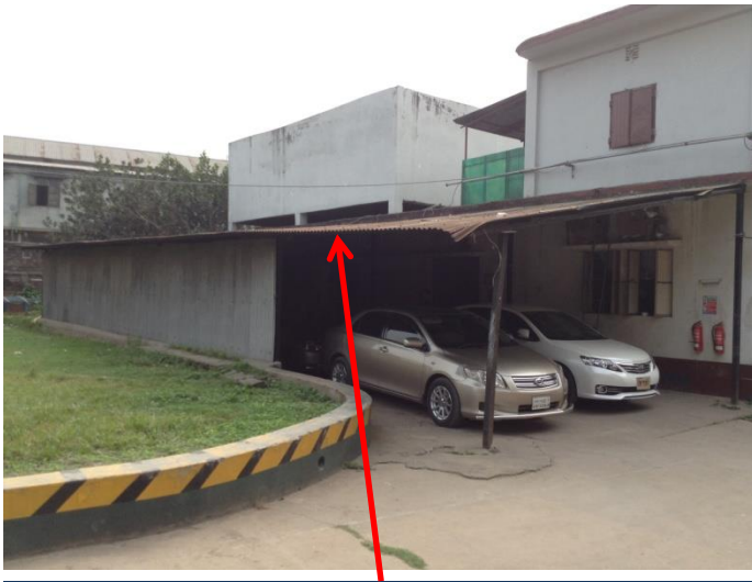
Additional tin shaded parking area appeared non-engineered
