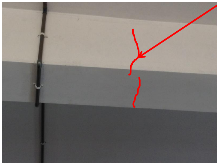
Cracking on beam at first floor
