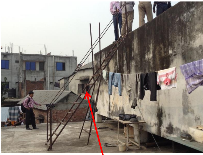
Non-engineered stair structure for water reservoir
