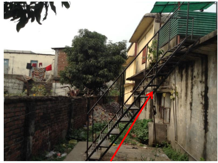
Non-engineered stair structure
