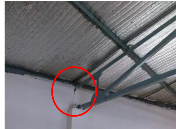
In general, no vertical truss members at bearing points
