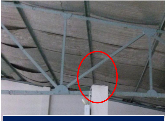
Supporting columns are NOT coincident with truss nodes
