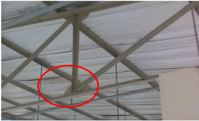
Very poor welds between truss members
