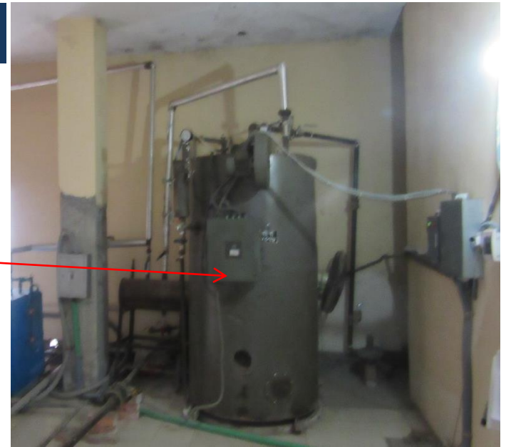
40-50KN boiler on 1 st floor
