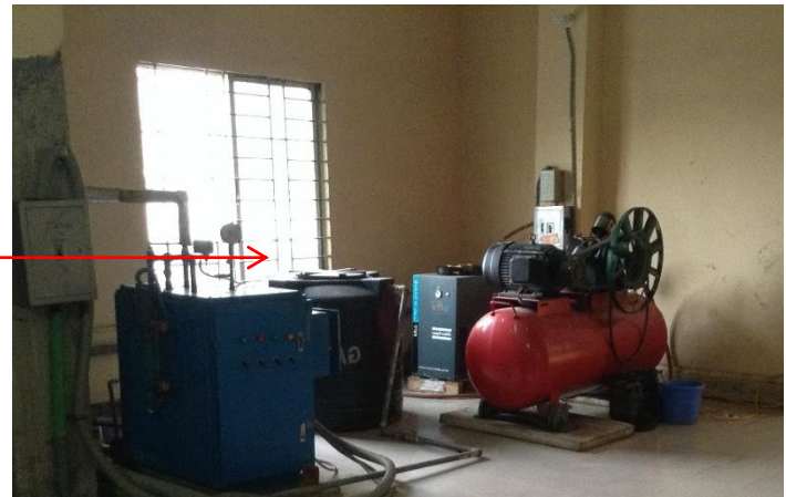
500L water tank on 1 st floor
