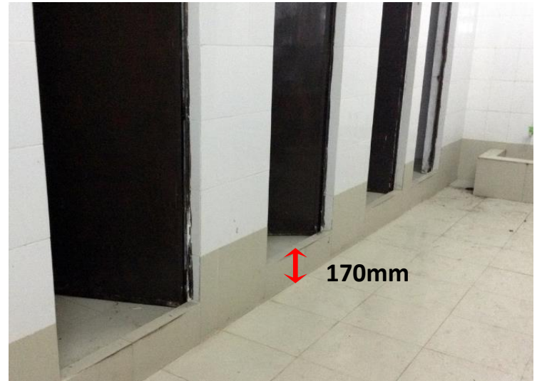
Build-ups observed in the toilet area.
