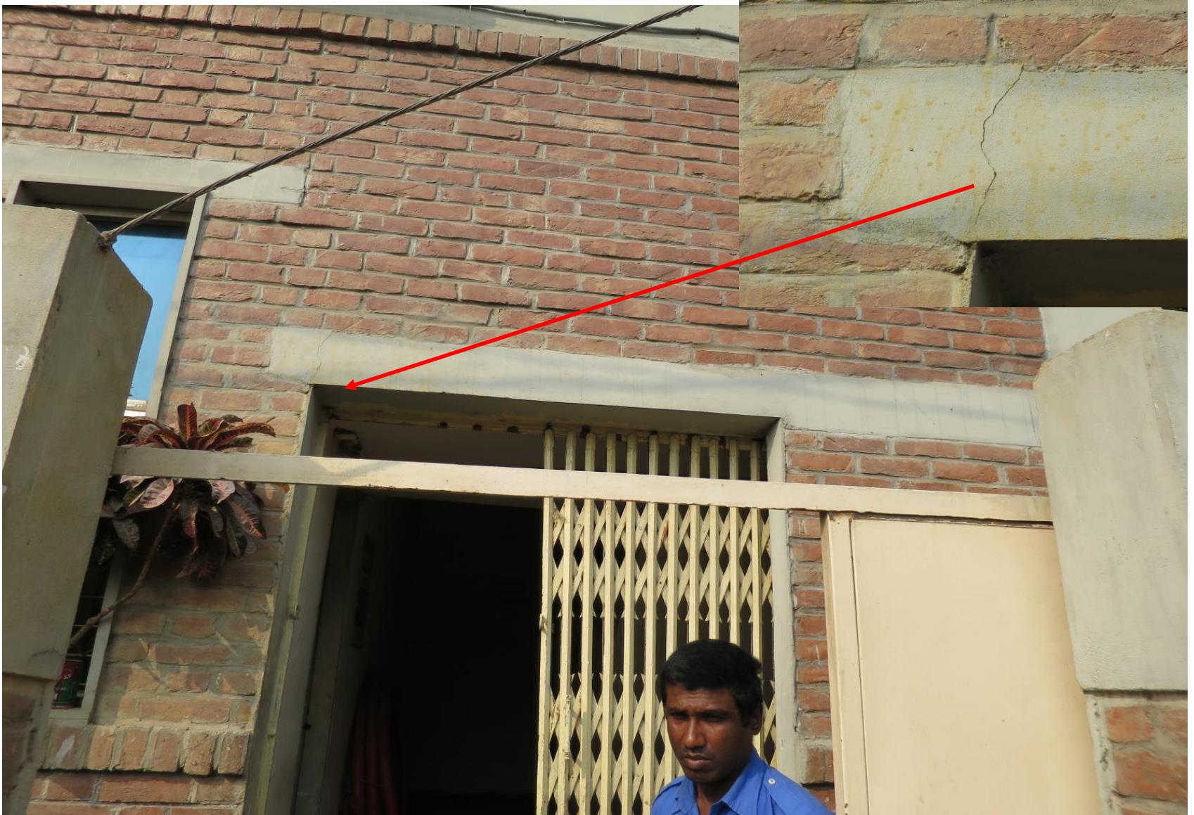
Cracking in the lintel over the door observed
