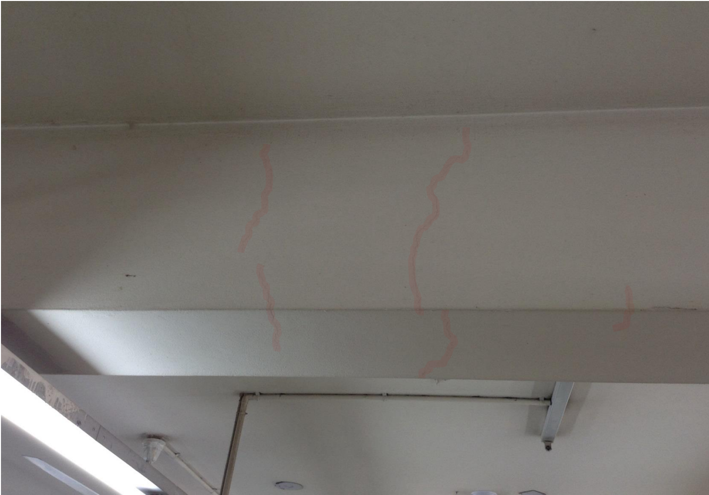
Minor cracks observed in 1 st and 2 nd floor beams
