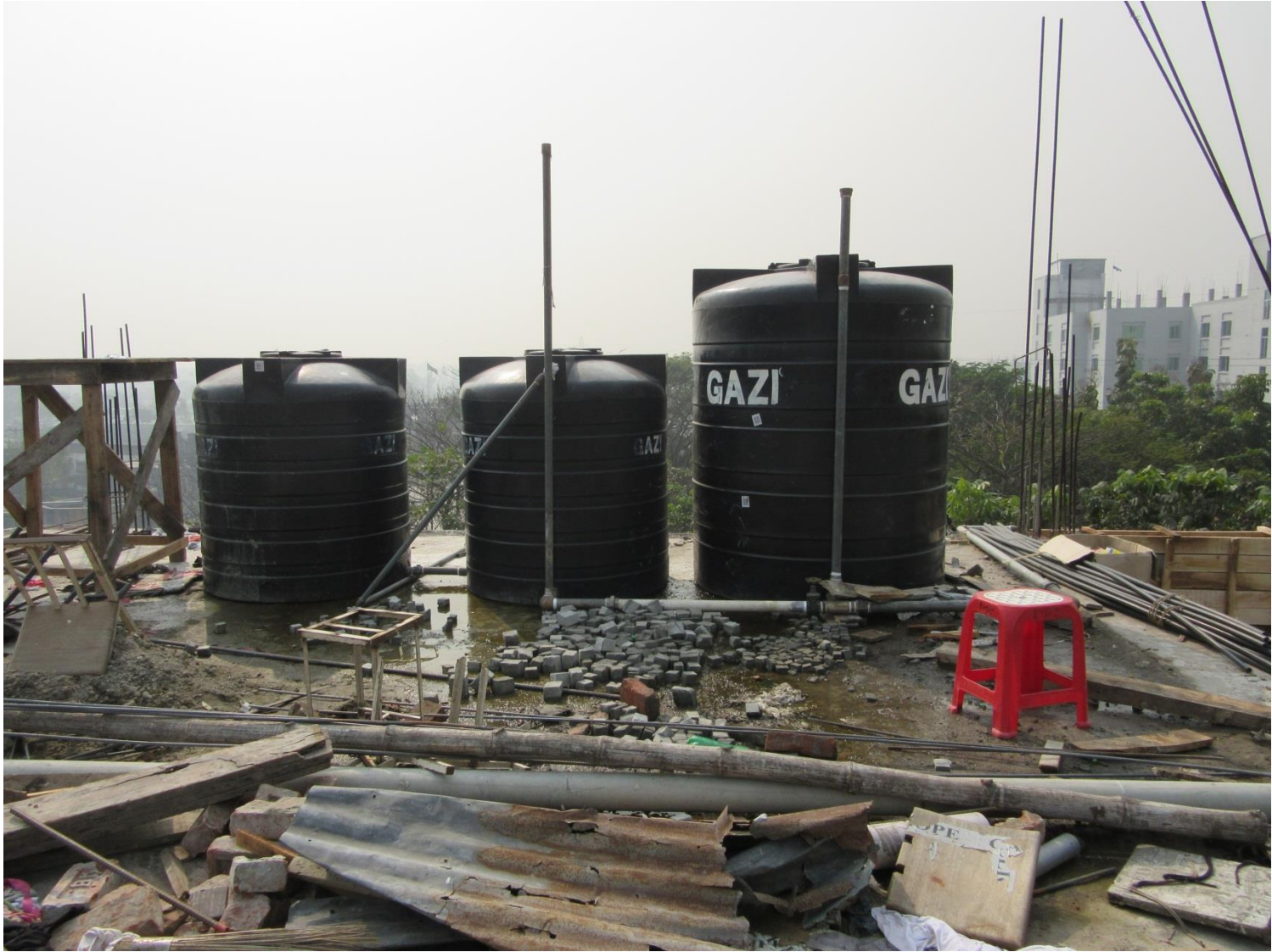
3 temporary storage tanks on the roof (2 x 1500 litres and 1 x 2000 litres)
