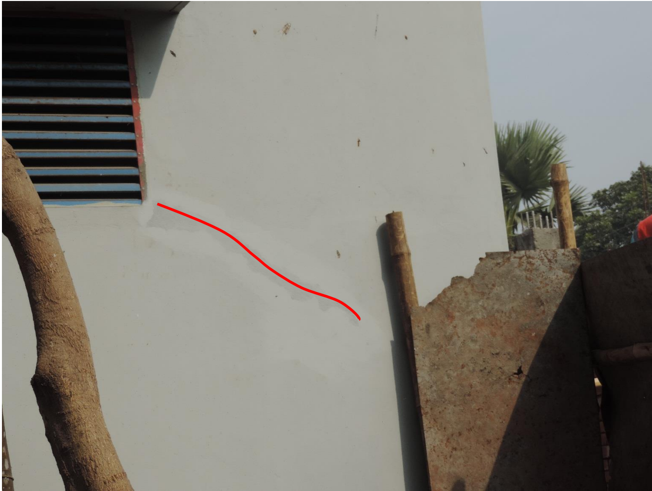
Crack is observed in external wall
