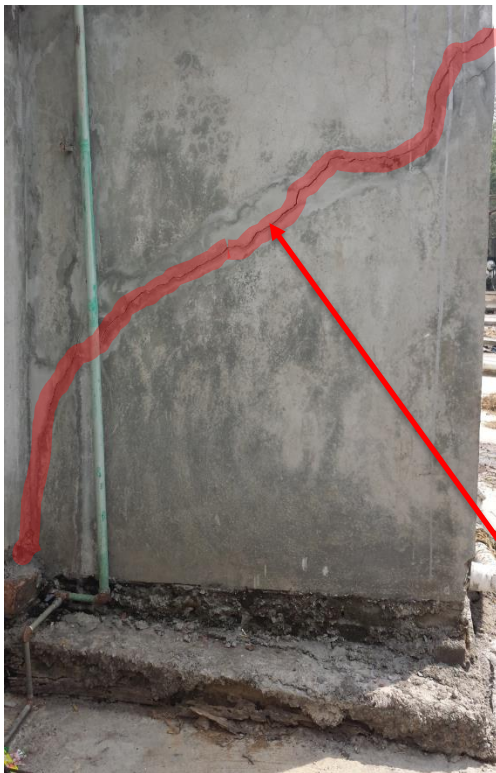
Crack observed in the external brick wall of the toilet area at Ground Floor.
