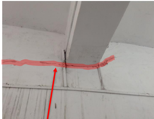
Crack on the partitions are observed in the toilet area .
