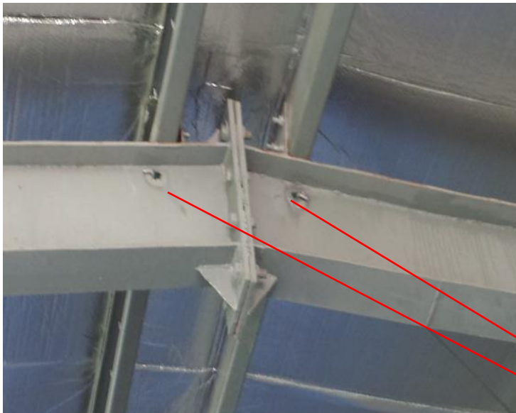
Holes observed in the web of the roof beams
