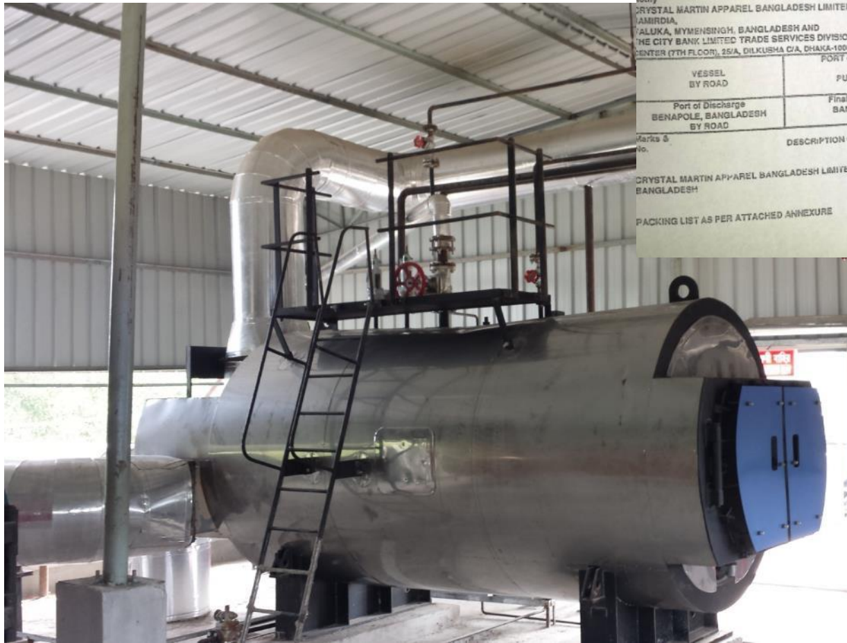
Boiler Machine weighs 150kN including water
