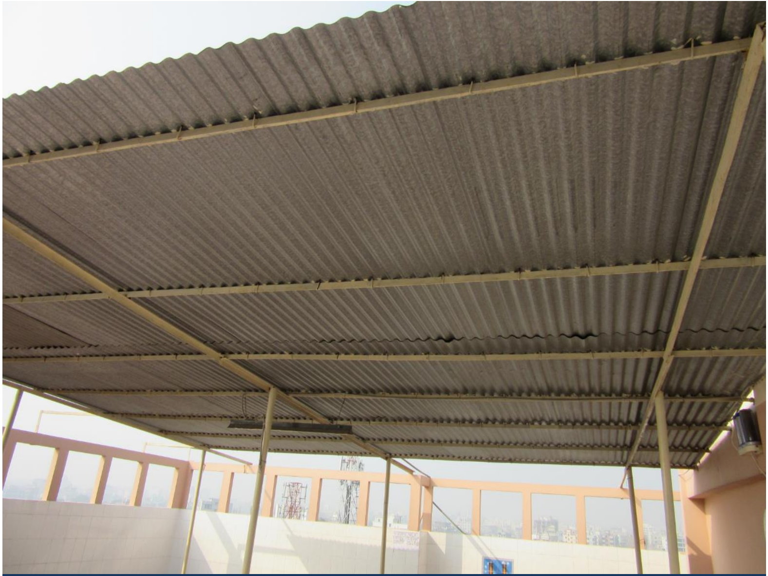
Apparently non-engineered steel shed over the building
