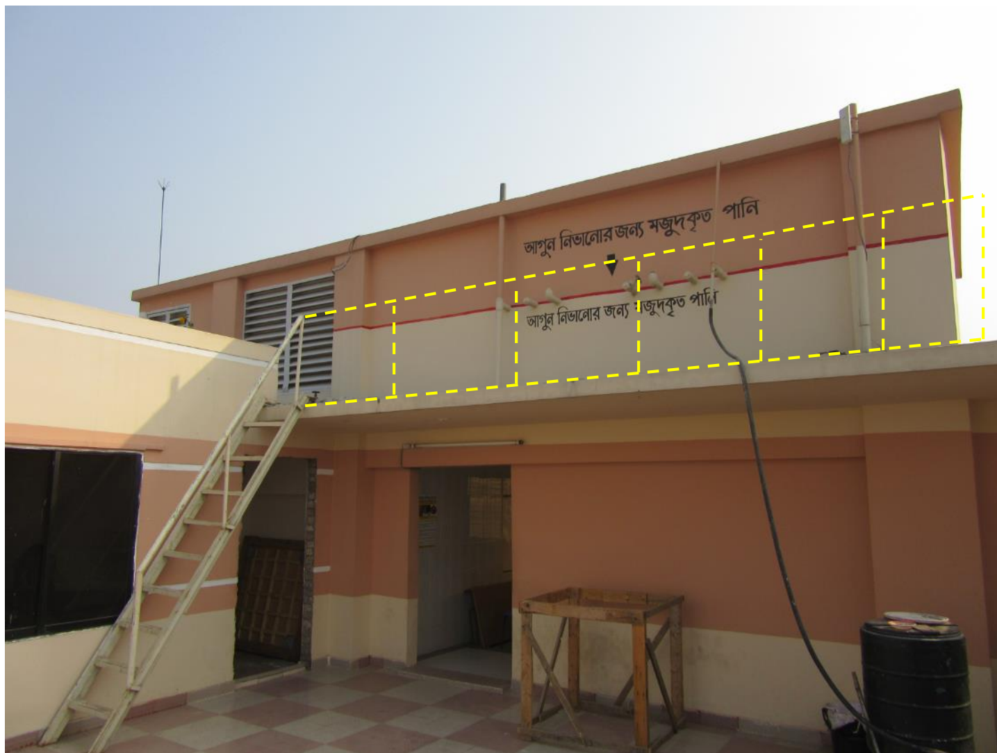
Lack of Safety rails on the roof and beside water tank
