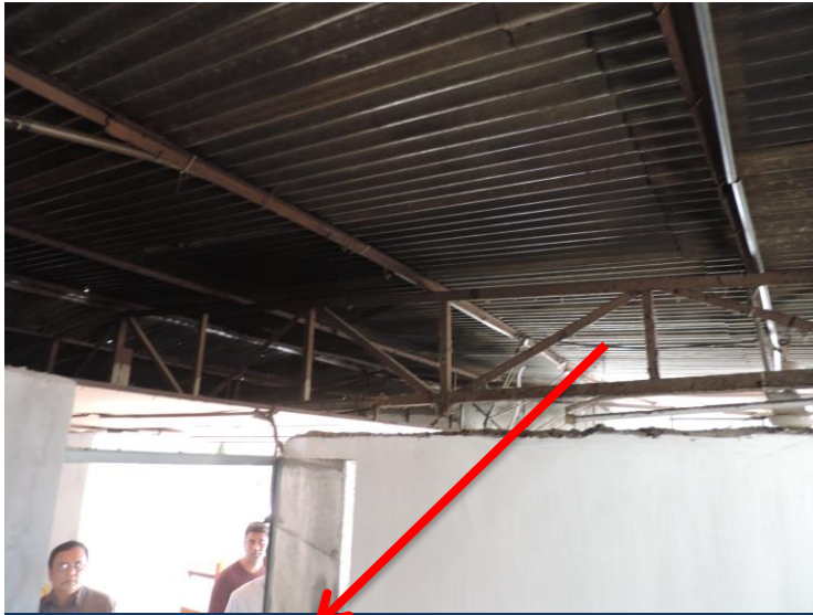
Poorly-constructed and non-engineered structure at roof top
