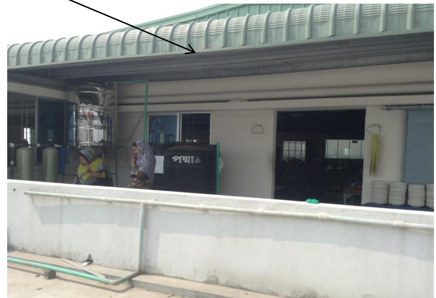
Steel structure not on permit drawing
