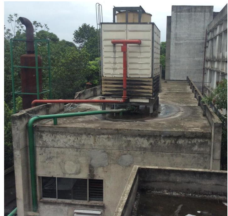
Roof of Generator Building, with no edge protection and water tanks positioned directly onto the slab
