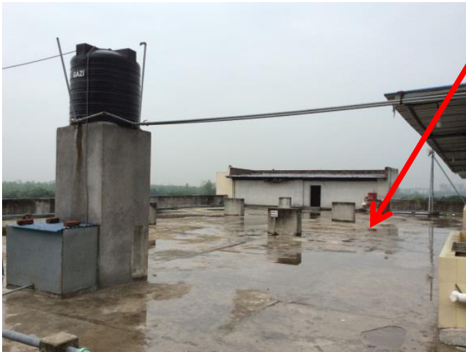
Roof of Main Building, with no clear drainage strategy
