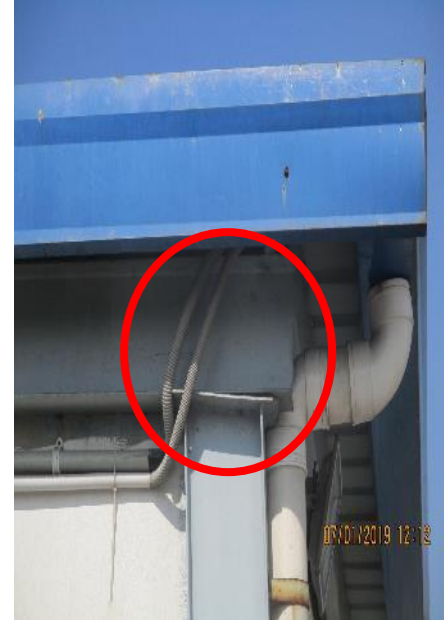
Improper welding connection between rafter and column
