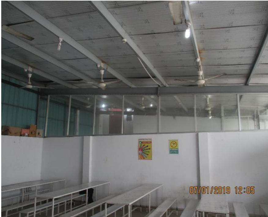
Steel frame (No vertical/Horizontal bracing)
