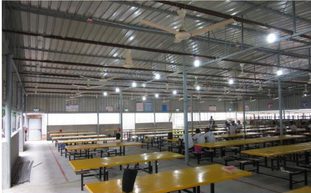
Canteen building with light steel truss structure in E-W direction, angle purlins N-S supported on 100mm Ø steel columns, with no stability cross-bracing
