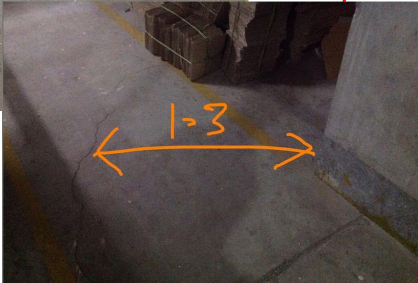
Cracking in basement slab
