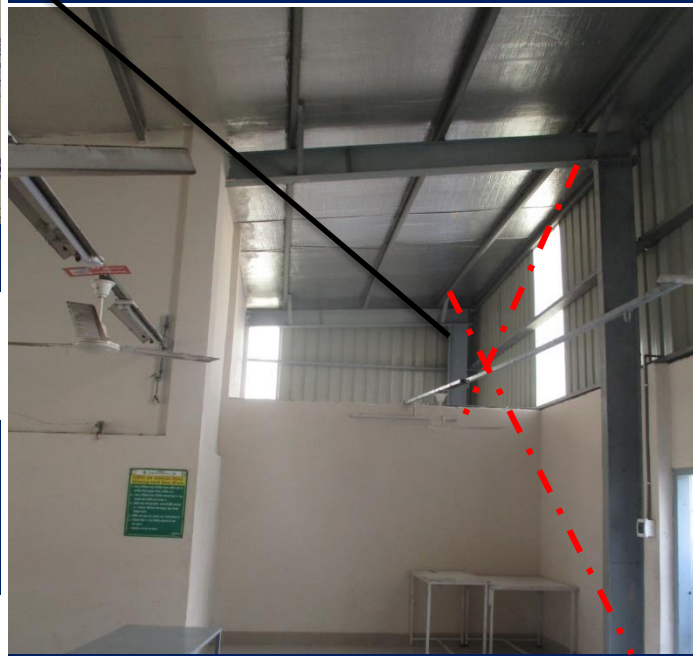
Vertical bracing not found in the marked location
