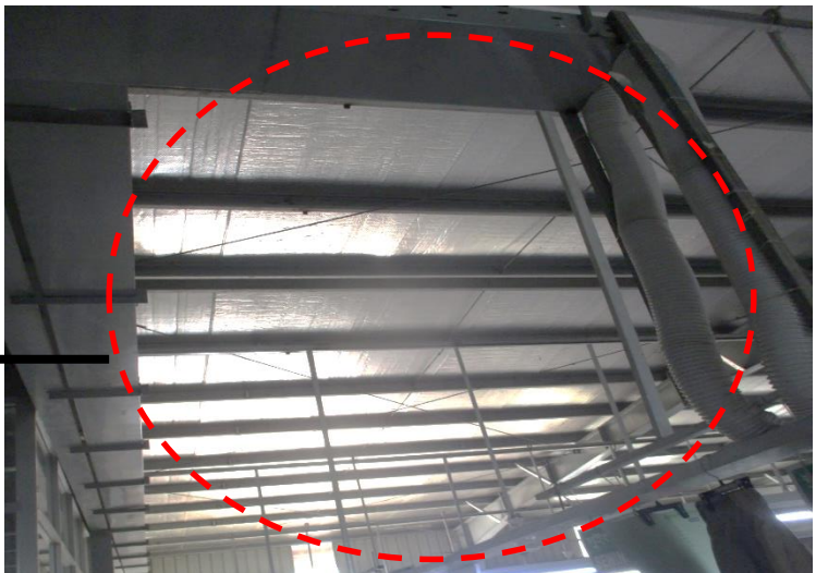
Onsite roof bracing location did not match with drawing
