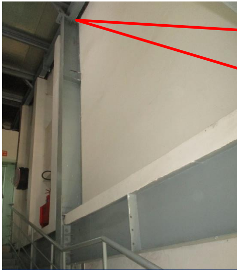
Connection of column and rafter was found different than drawing
