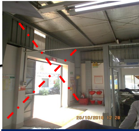
Vertical bracing not found according to the drawing
