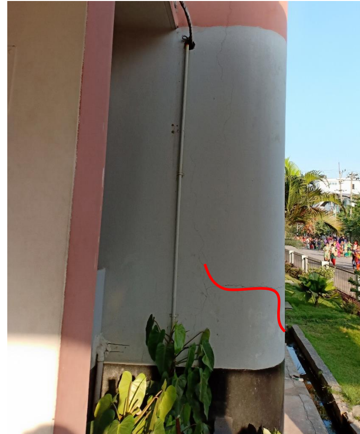
Minor cracks on wall
