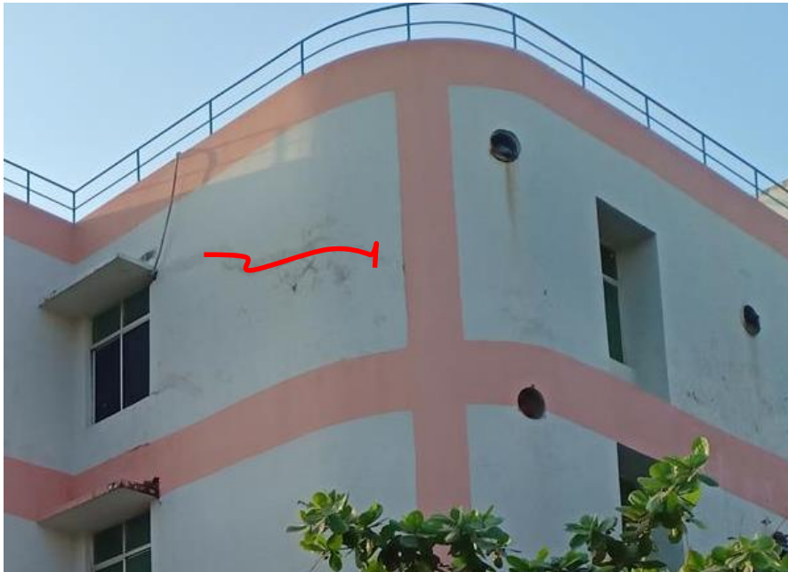
Cracks at North façade
