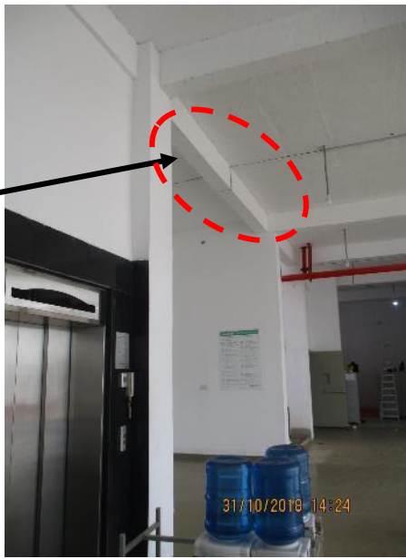
1st floor beam which was suppose to be retrofitted
