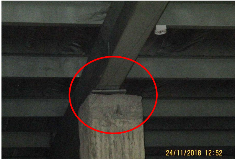
Apparently inadequate bearing area in joint
