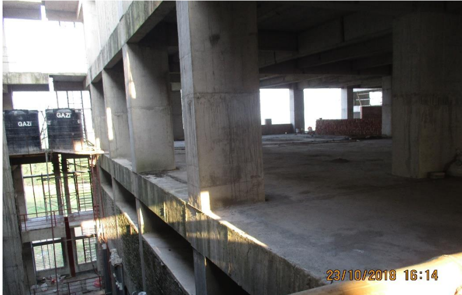
Parapet missing in Garments Building
