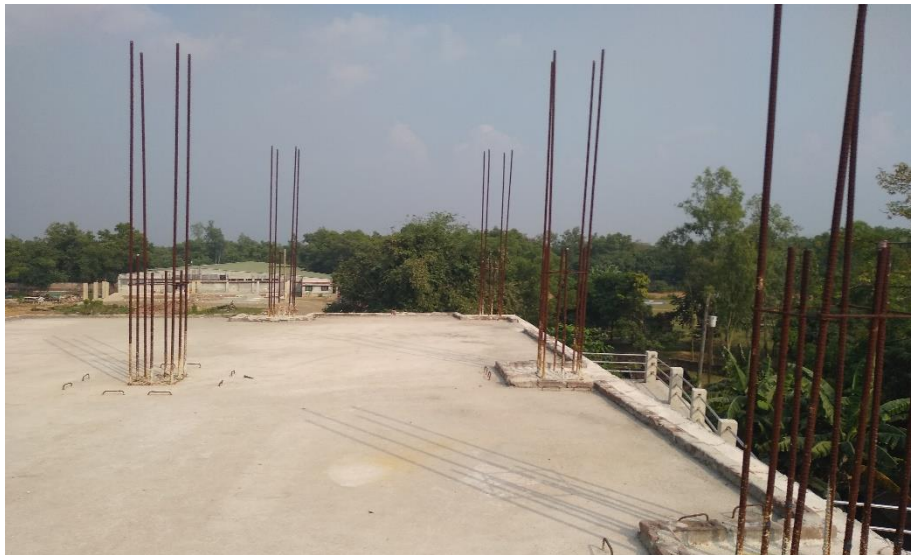
Parapet missing & Exposed rebar at Utility Building
