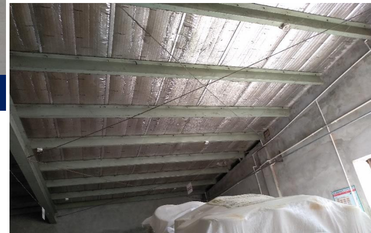
Loose cable bracing
