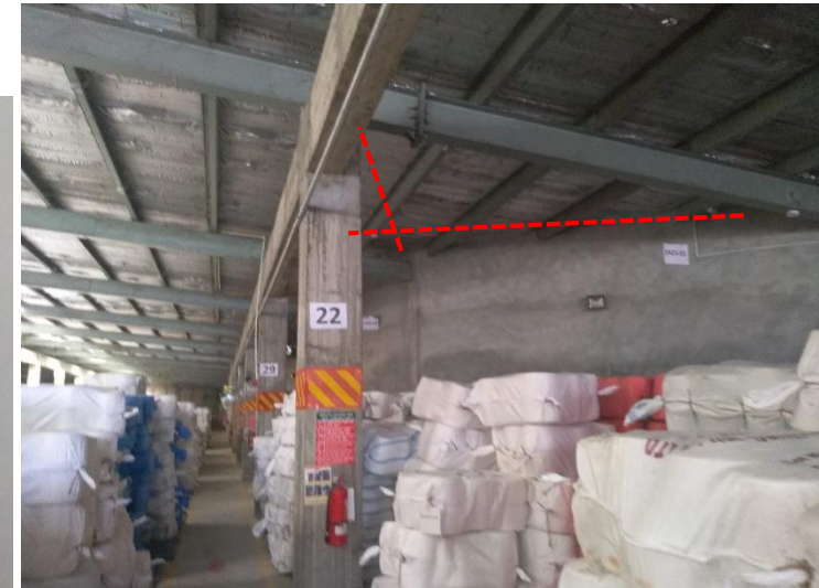
Missing roof bracing
