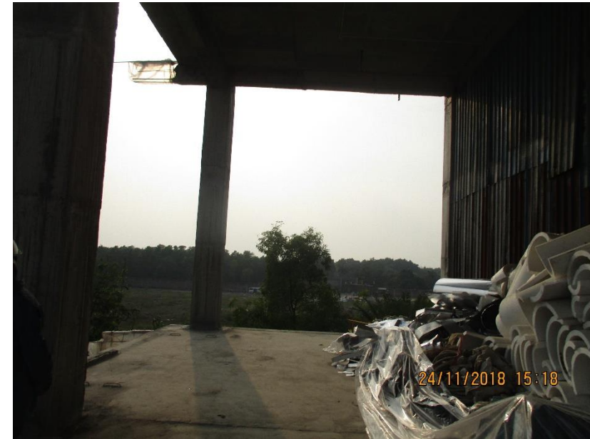
Parapet missing at Generator & Chiller Building
