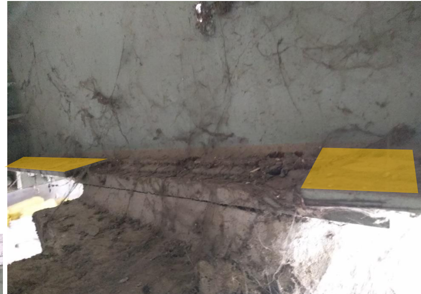
Flange discontinued joint connection
