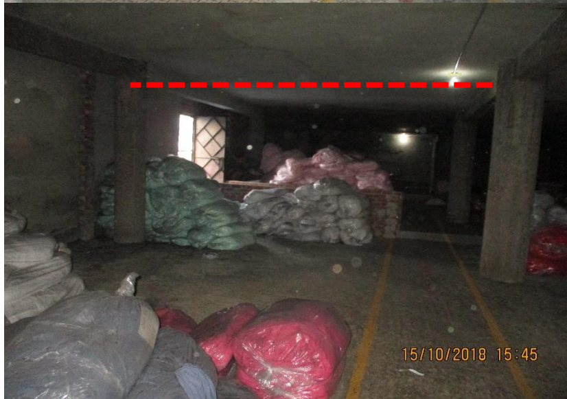
Missing beams in short direction
