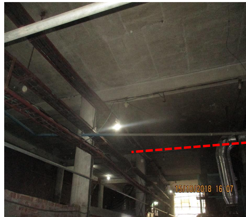
Missing beam in short direction
