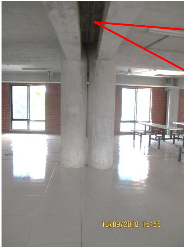
Gap at expansion joint covered with mortar and tiles
