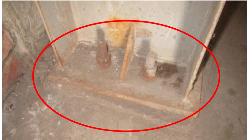
Corrosion was observed at joint of steel column and pedestal column
