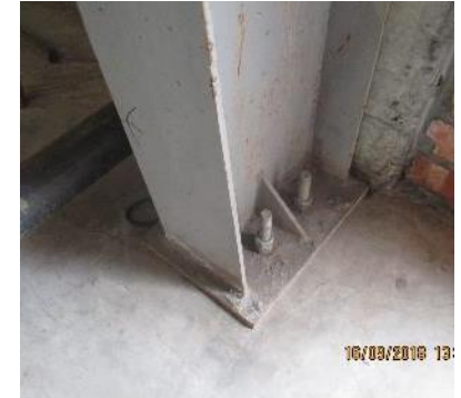
Bolted connection between pedestal column and steel column
