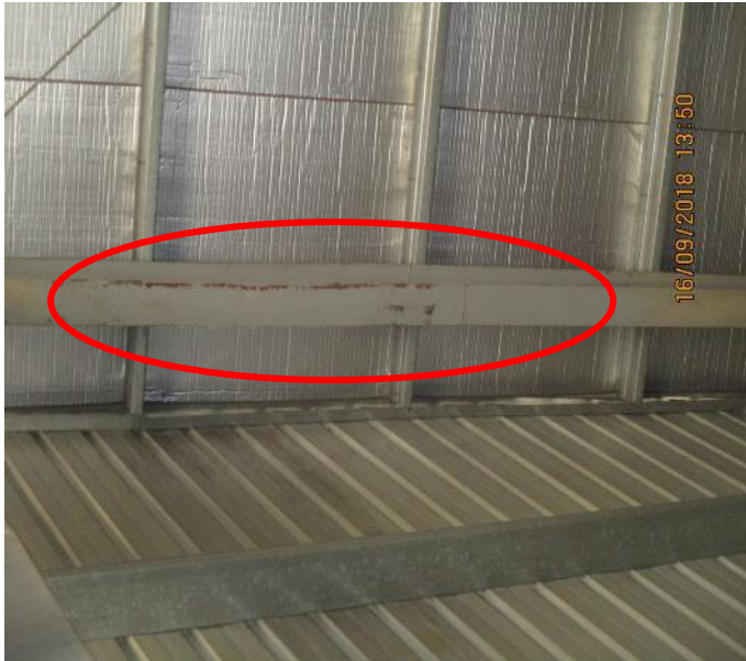
Corrosion was observed at rafter
