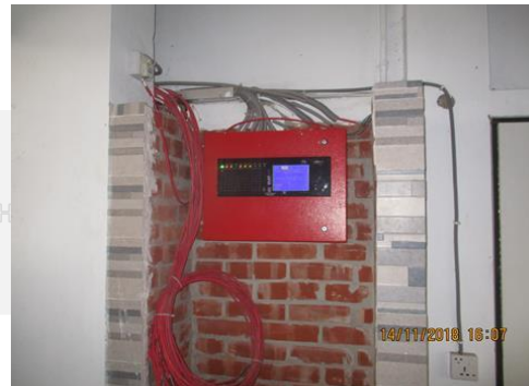
Fire Alarm control panel
