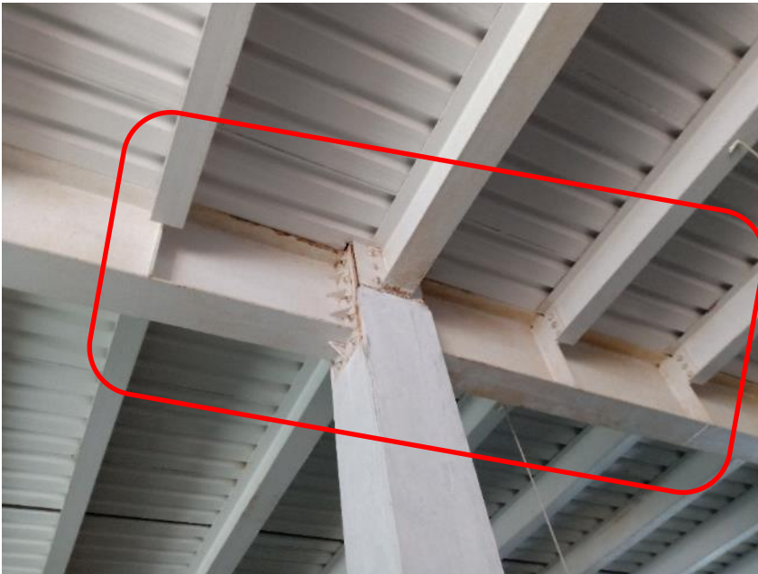
Corrosion at beam-column joint
