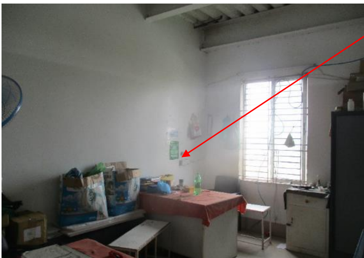
Vertical Bracing missing
