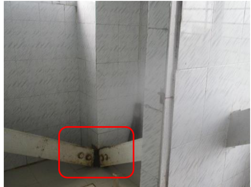
Corrosion at bracing connection
