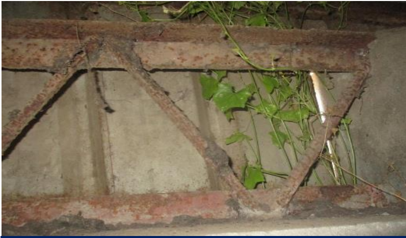
Extensive corrosion observed in truss member
