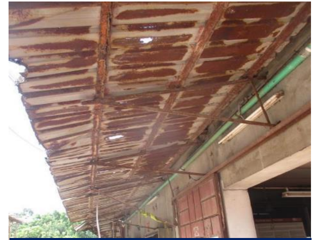
Extreme Corrosion observed in canopy
