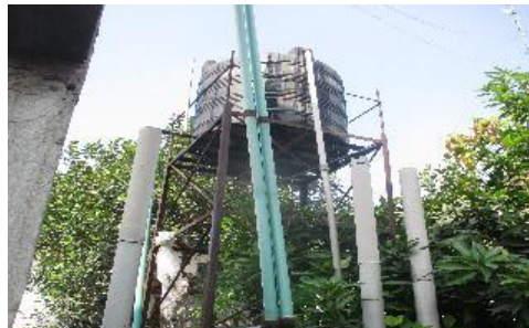
2000 litre water tank on steel frame over women toilet roof top
