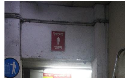
Deflection of roof slab of men's toilet
