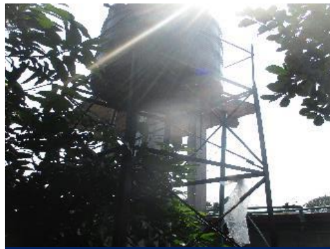
2000 litre water tank on steel frame over men toilet roof top
