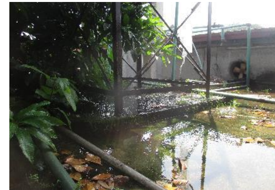
Water clogging observed over roof top of men's toilet
