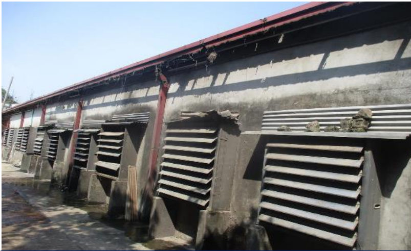
Extensive corrosion observed in gutter
