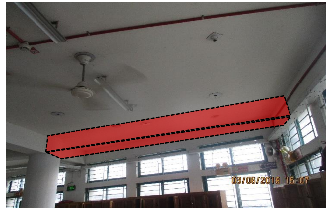
Location of the missing beam
