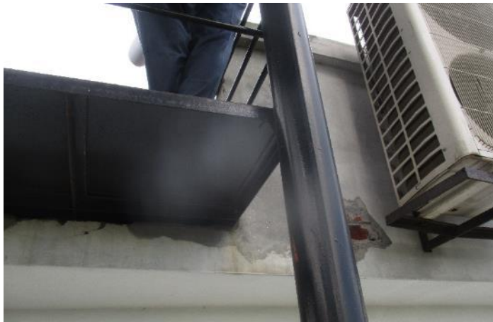
Stair landing Poorly connected with office building
