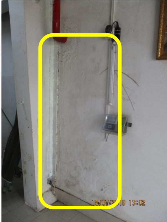
Dampness on periphery wall
