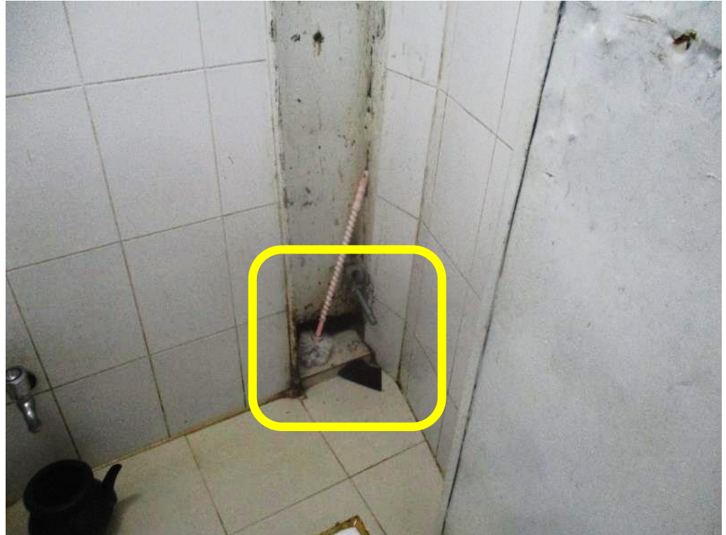
Corrosion at column base inside toilet zone
