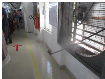
Loose vertical bracing
