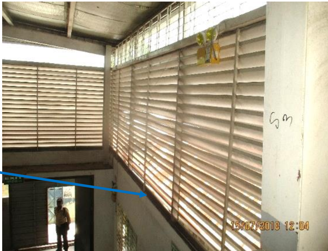
End beam missing at East stair
