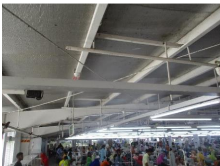
Loose roof bracing
