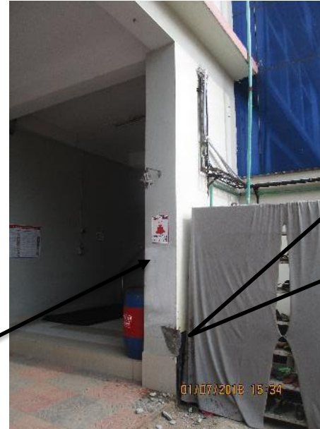
Mixture of stone & brick aggregate was found in the marked column
