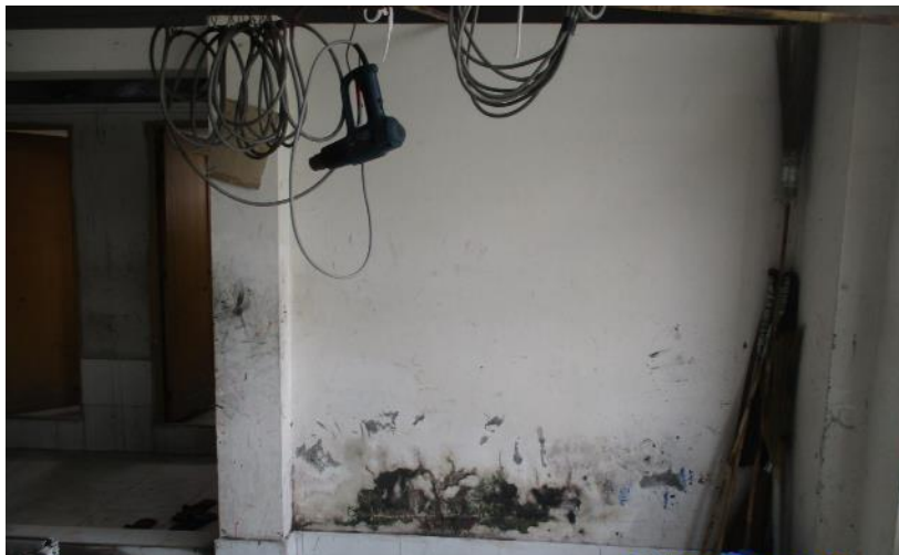
Extensive dampness was observed on masonry walls of toilet area on different floors
