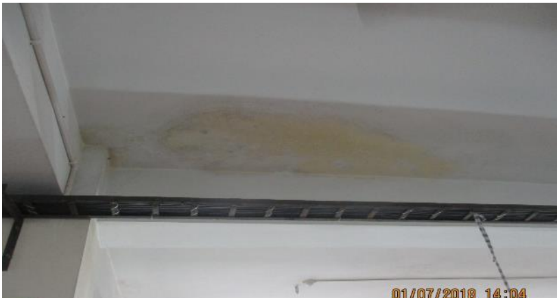
Dampness was observed on roof slab of top floor
