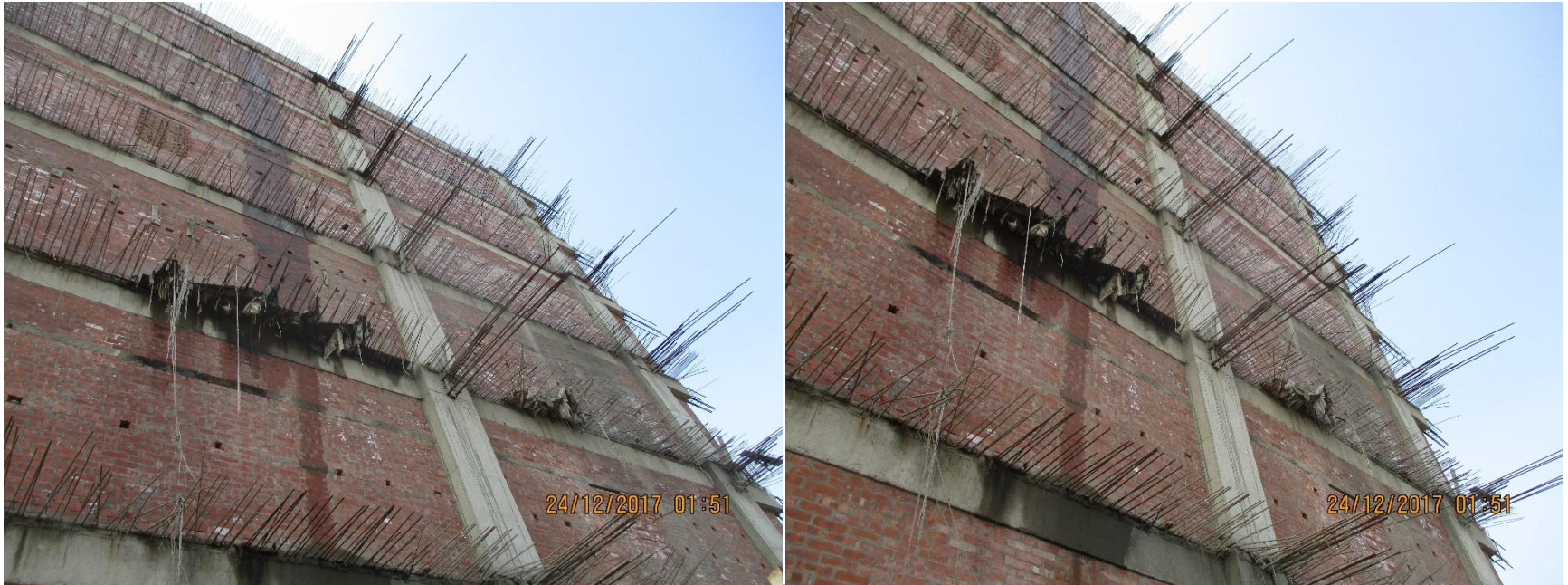
Rebar exposed to weather
