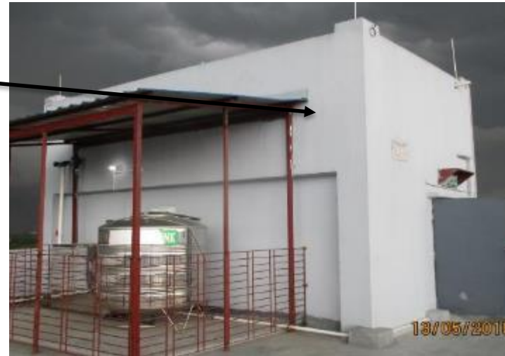
Water tank (6.8mx3.1mx1.4m)
