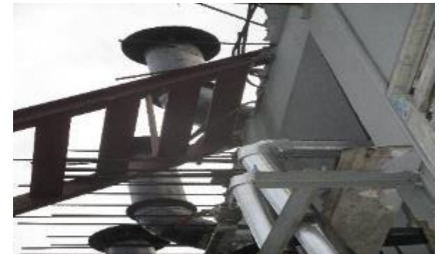
Stair end resting on generator room slab
