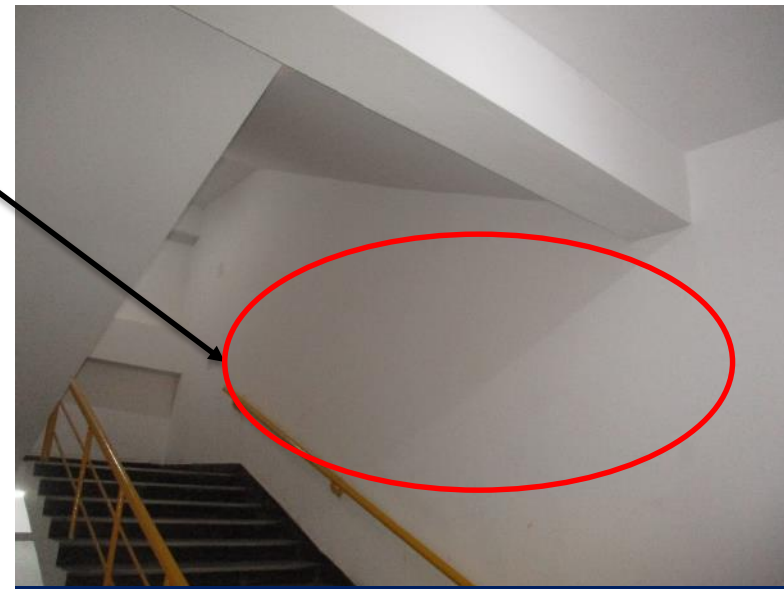
The marked beam was not found on north-west side stair case
