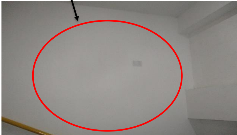
The marked beam was not found on south-west side stair case
