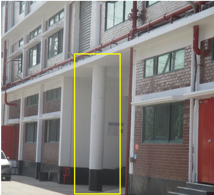
Columns at loading bay are susceptible to impact loading from vehicles.
