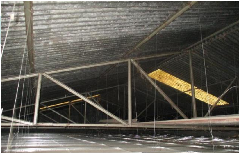
Roof bracing was missing
