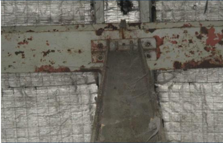
Corrosion on column rafter joint.
