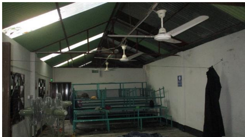
The support condition of the truss was appeared to be non-engineered and inadequate
