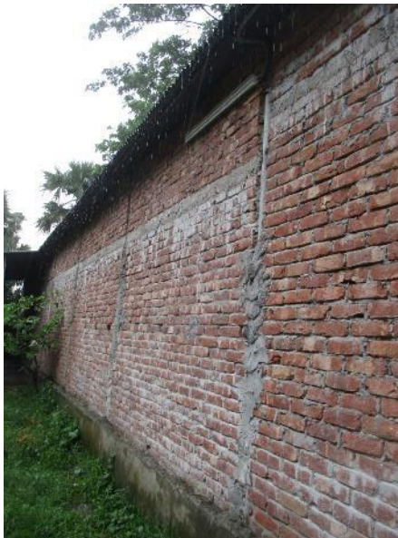
Truss has been found supported with steel pipe on north side and the welded joint was used as a connection
