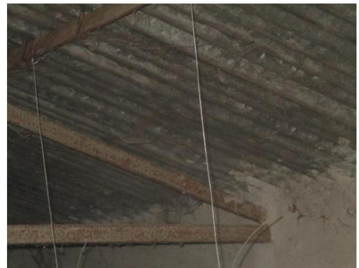
Truss has been found supported with brick wall on south side. It appears to be a non engineered connection.
