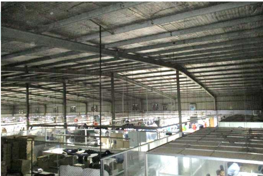
No roof bracing
