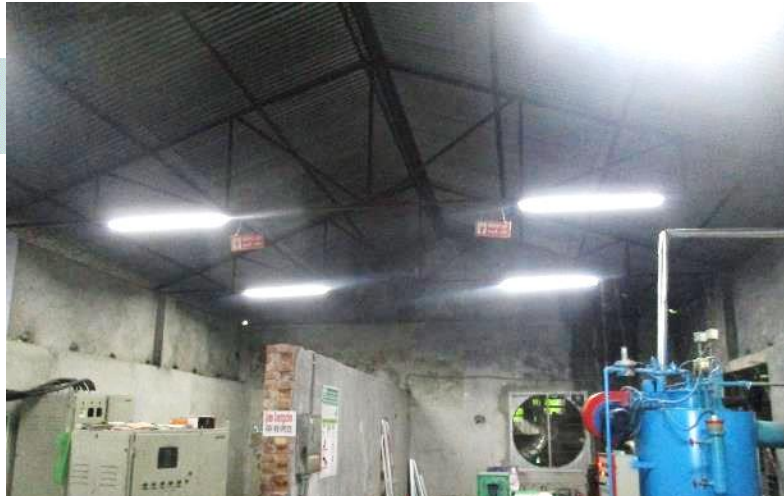
Roof truss system with out any bracing and supported by brick wall.
