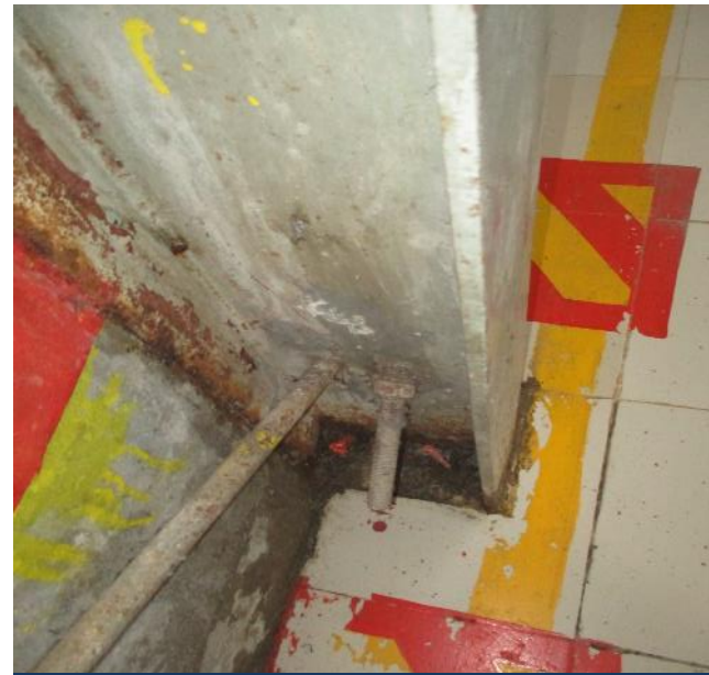
Corrosion on column in front of north east toilet area
