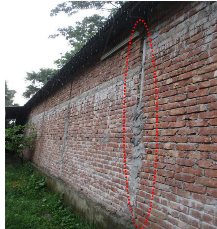
Steel pipe support was found on east side in-place of brick wall.
