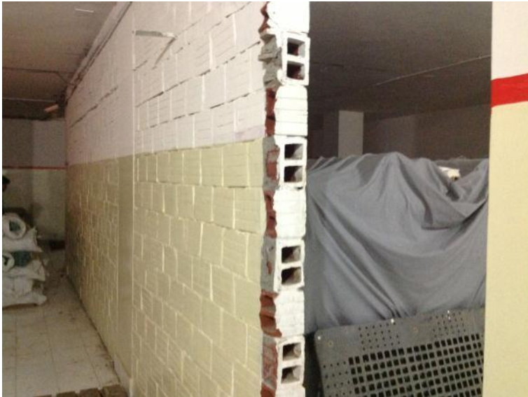
Slender wall without end restraint. Vulnerable to horizontal impact when moving material or machinery.
