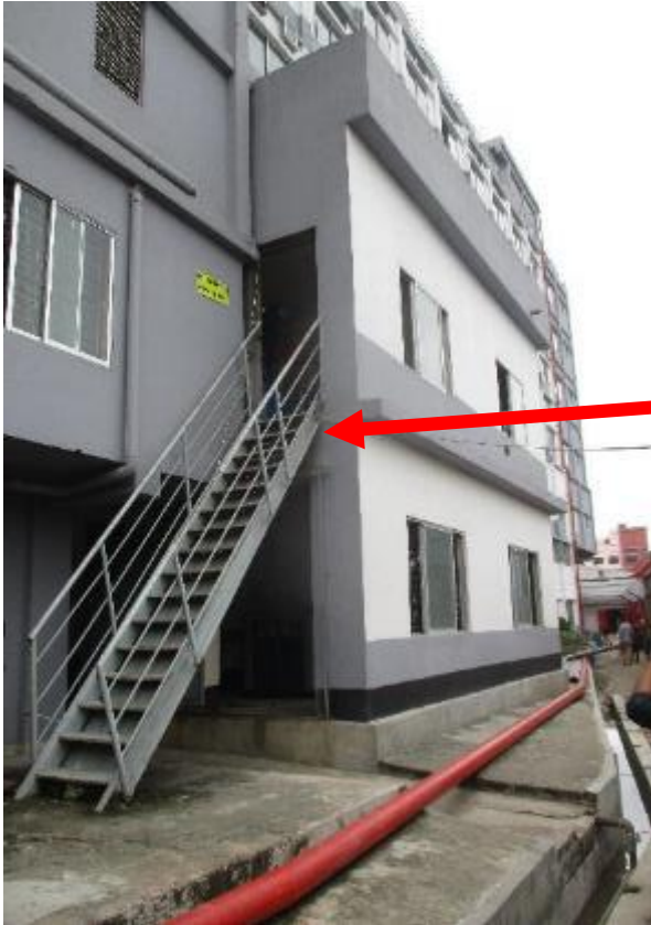
Non-engineered steel stair at the east side of Utility building.
