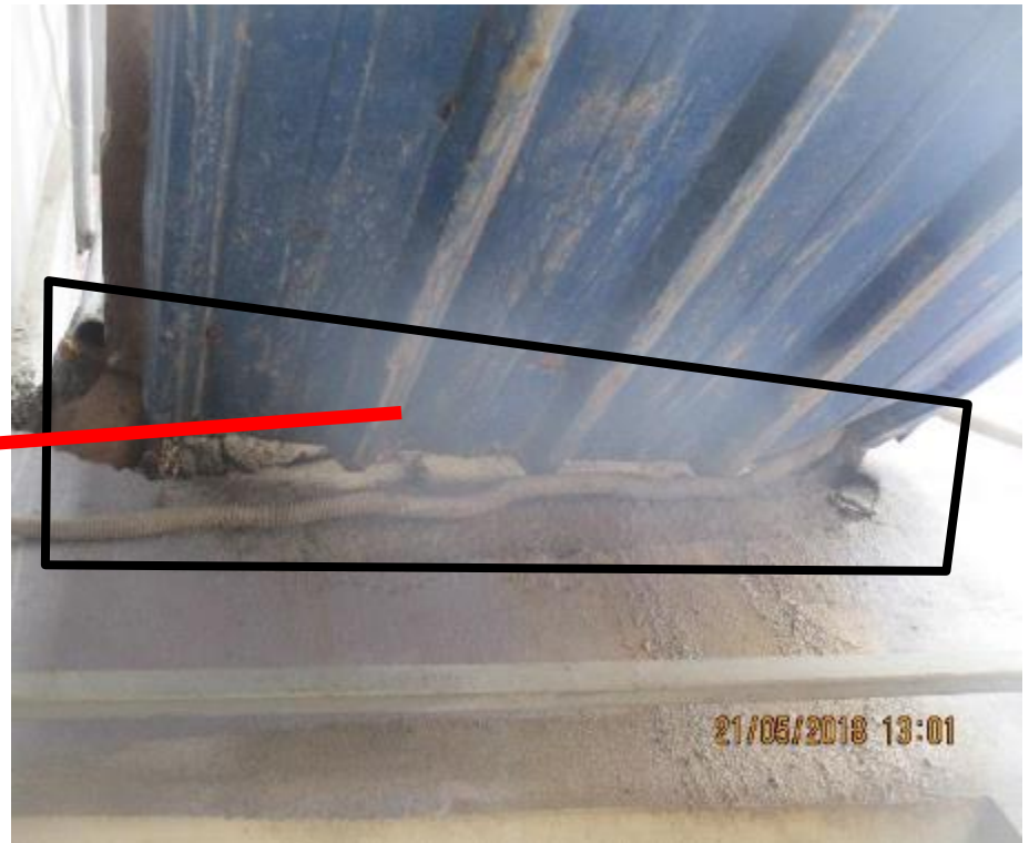
Steel stair poorly connected with slab. Factory engineer is required to check the stability of the steel stair.
