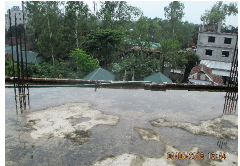
No obvious drainage system was observed
