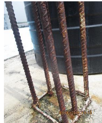
Corrosion observed on exposed rebar
