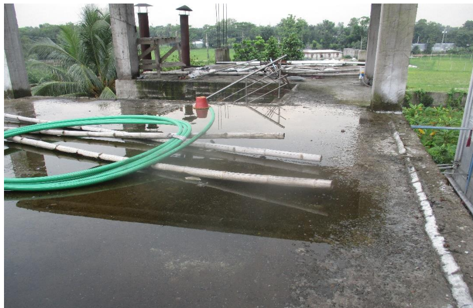
Stagnant water due to improper drainage system
