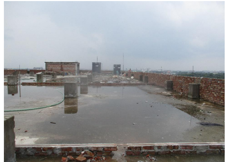
Stagnant water on roof
