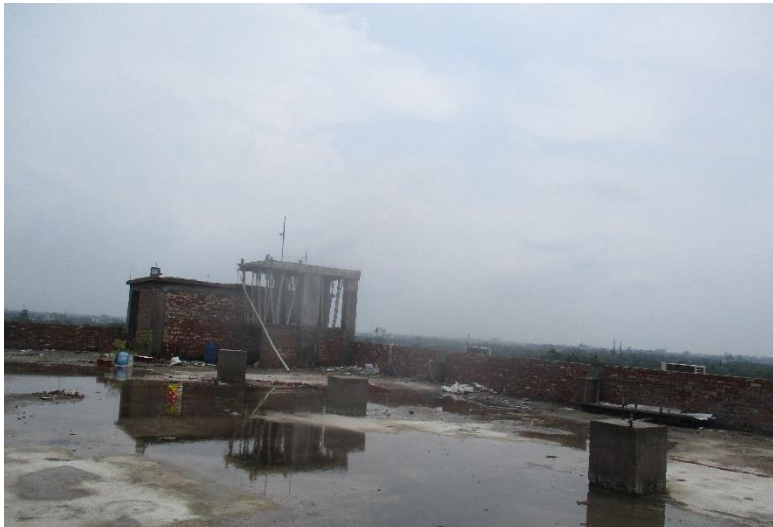
Stagnant water on roof
