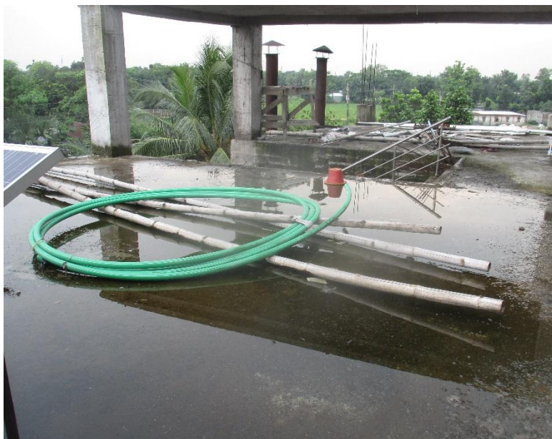
Stagnant water on roof
