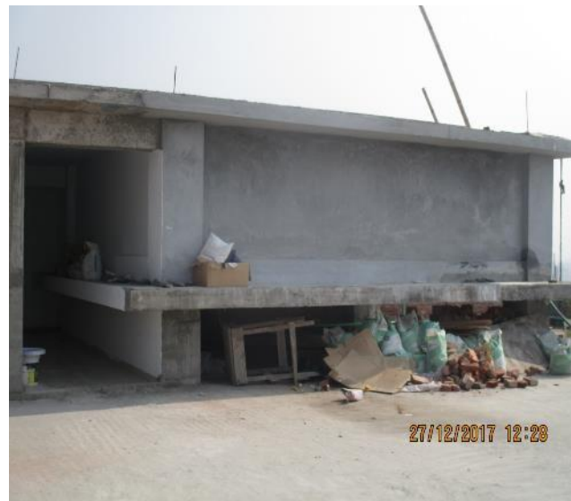
RC water tank on roof top having capacity 50000 liter
