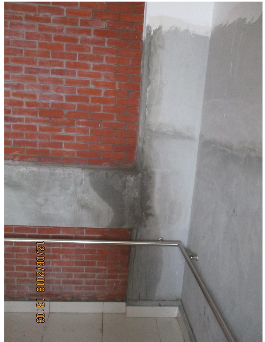
Dampness on structural member
