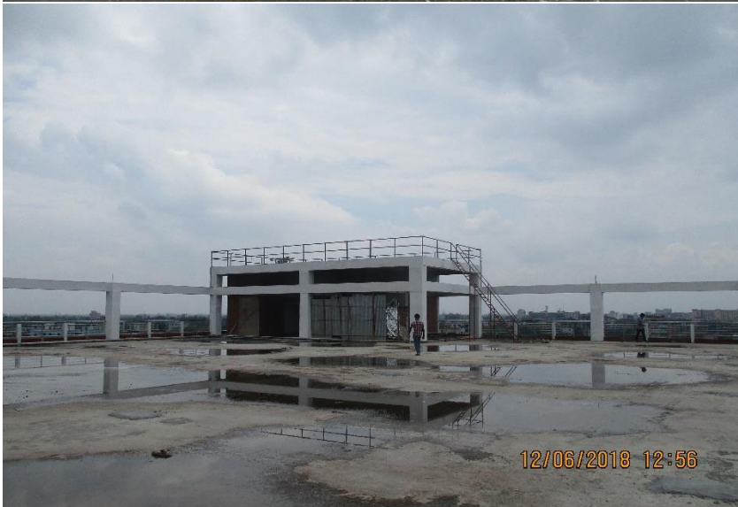
Poor water drainage system
