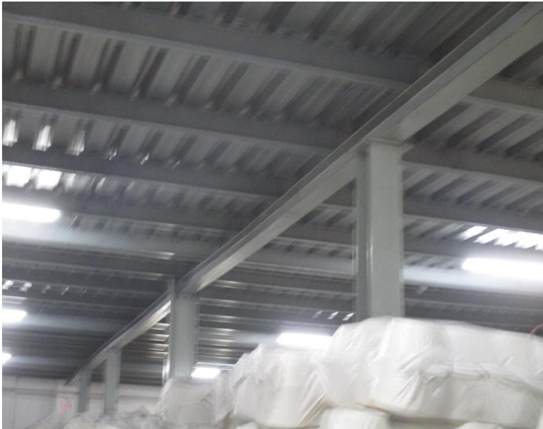
Deflection of main beams
