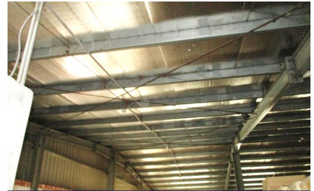
Sagging of cable bracings
