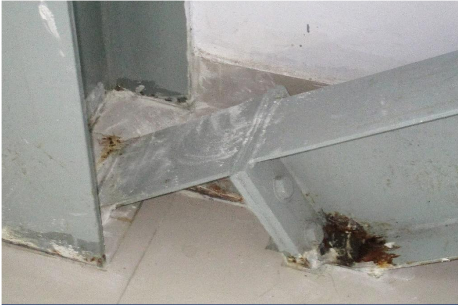
Corrosion observed at the joint of column and bracing.
