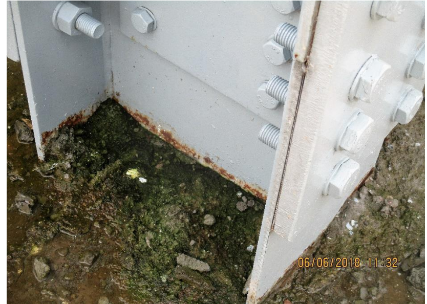
Corrosion was observed on steel column at roof top.
