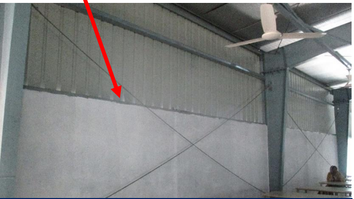
Only cable bracing was found in grid 1B-1C & 1C-1D but no compression strut was observed.
