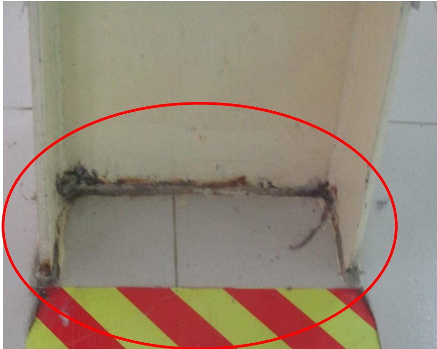
Corrosion was observed at joint of deck slab and steel column of 1 st floor in production areas.
