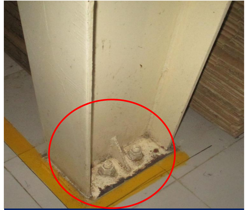
Corrosion was observed at joint of pedestal column and steel column.
