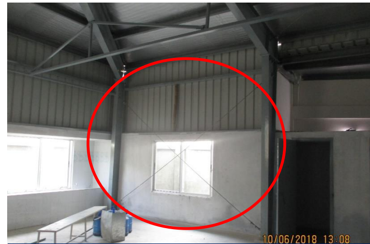
Loosely tied vertical cable bracing at west side
