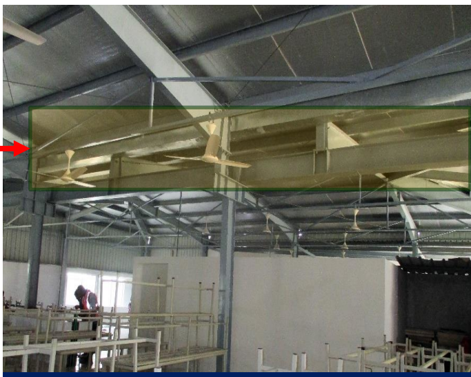
No column bracing was found on site in grid 5B-5C, 5C-5D, 7A'-7B' & 7B'-7C'
