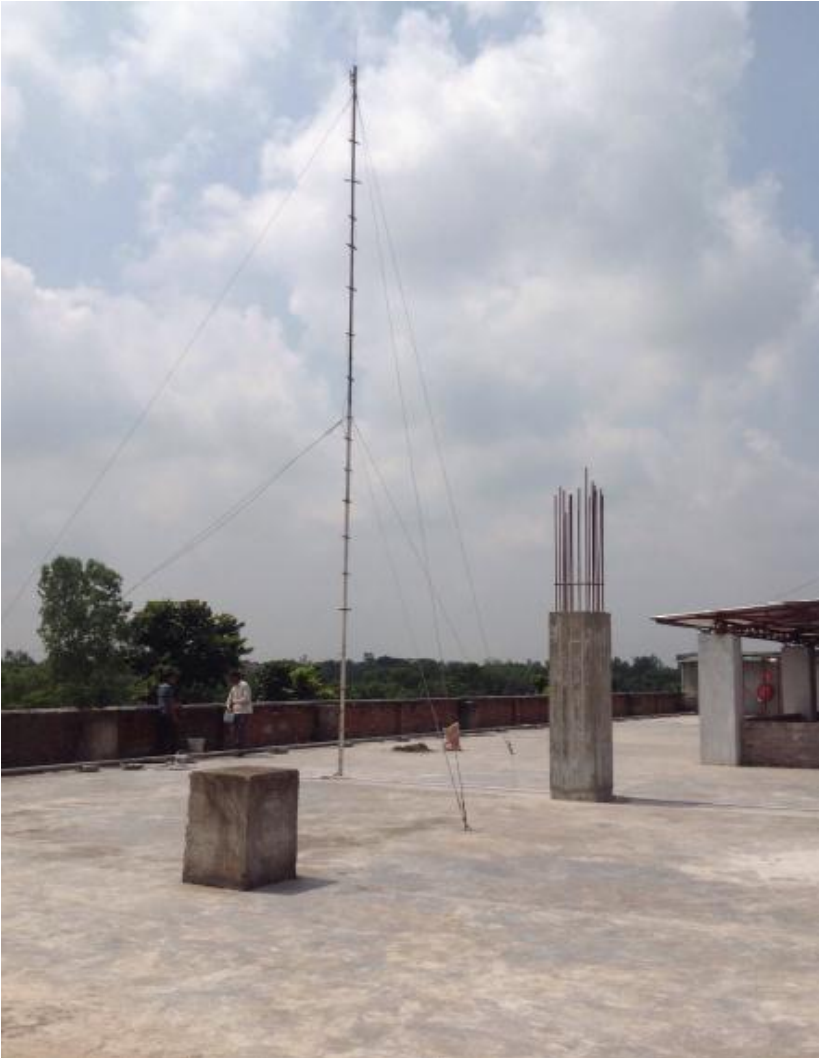
Antenna at roof level
