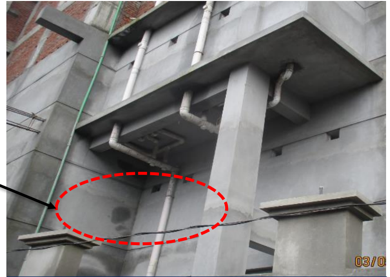
The marked beam was absent on 1 st floor under south side toilet zone but the beam was shown in beam layout.
