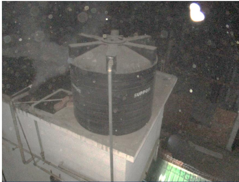
5000 ltr. water tank above boiler building
