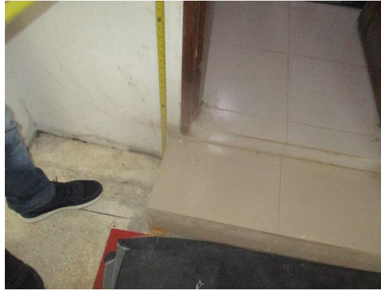
Toilet area with build up
