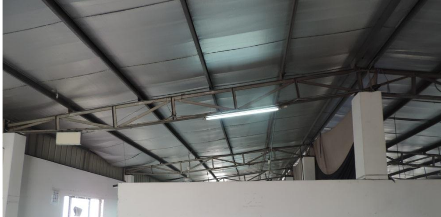
Lack of horizontal bracing in roof
