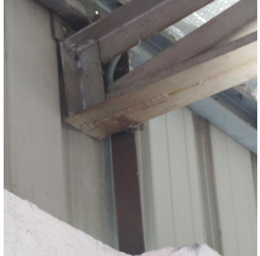
Non-engineered connection to column
