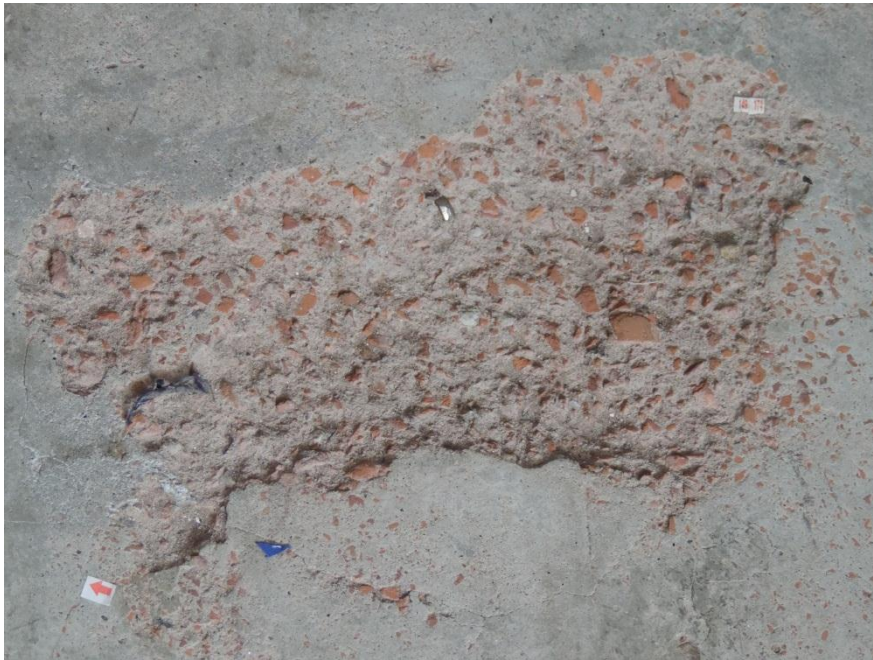
Brick aggregate in slab
