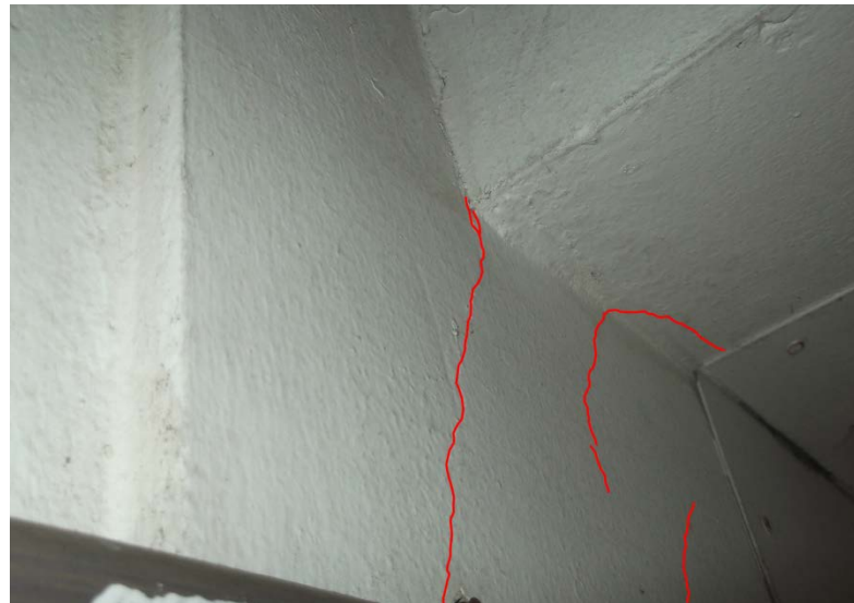
Cracks in beams / columns
