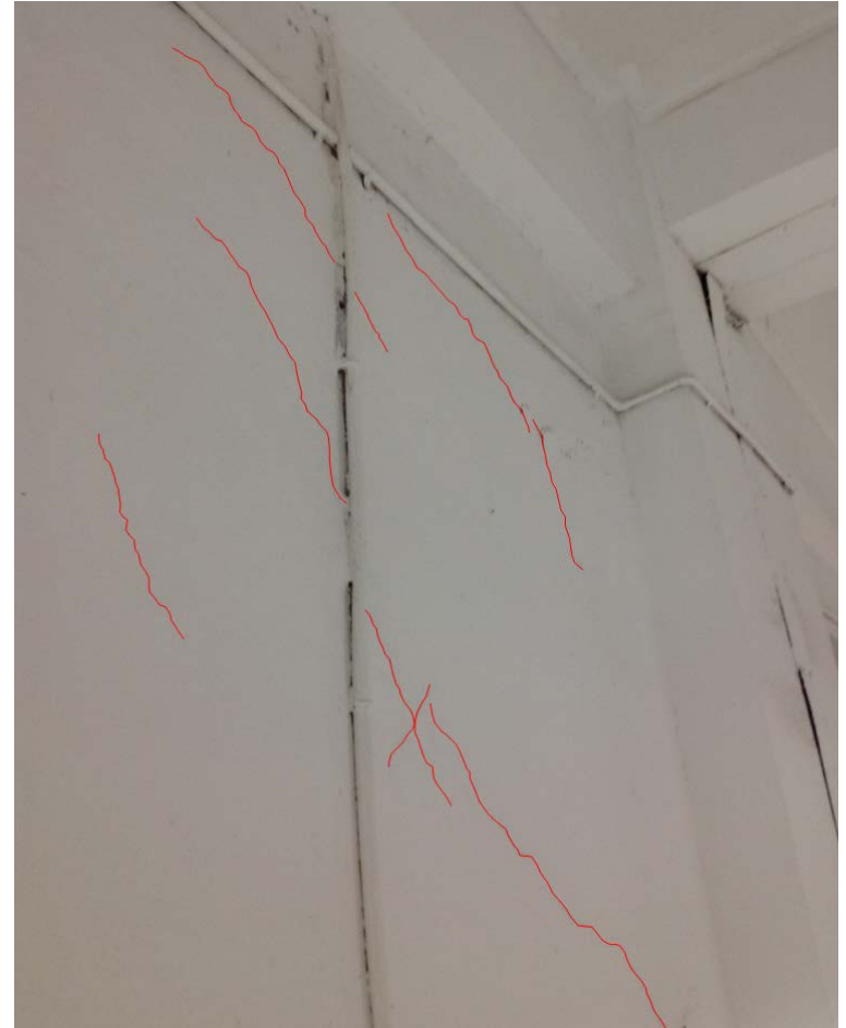
Crack in partitions 1 st floor
