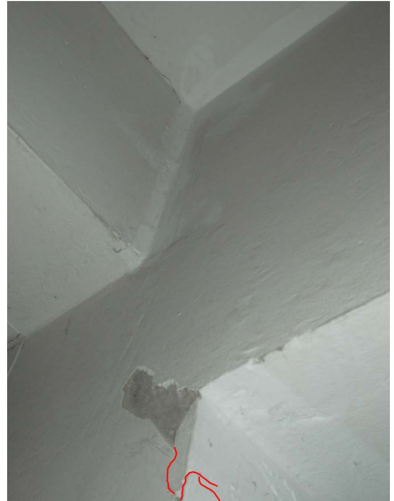
Cracks at the junction of the beam / column
