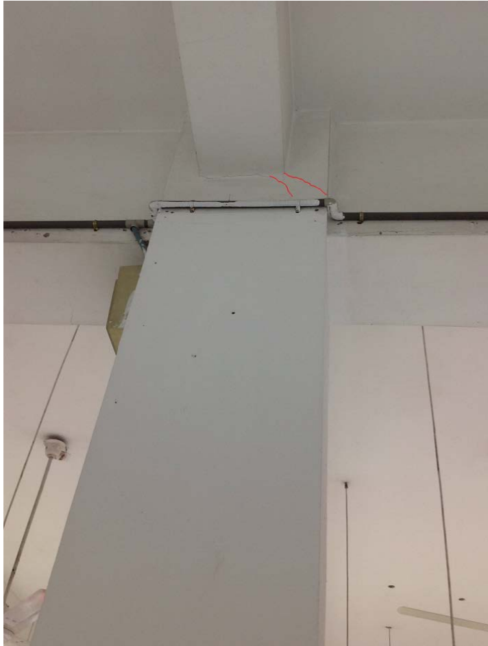
Crack in column 1 st floor
