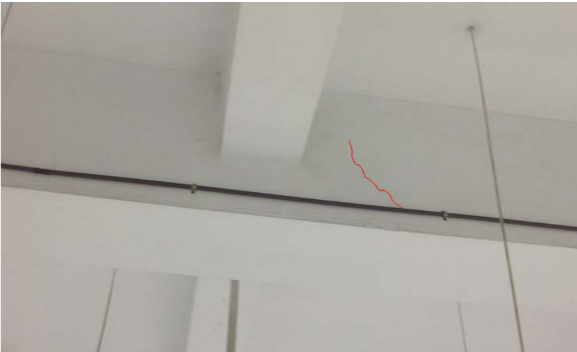
Crack in beam – u/side 2 nd floor
