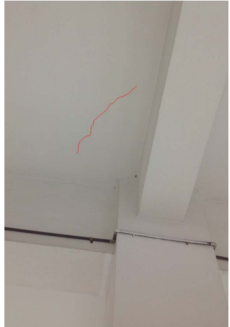
Crack in slab u/side 2 nd floor
