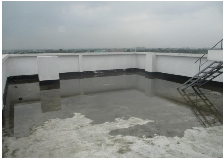
Stagnant water on roof
