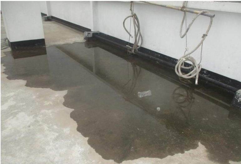
Stagnant water on roof
