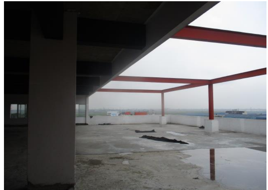
Stagnant water on 5 th floor
