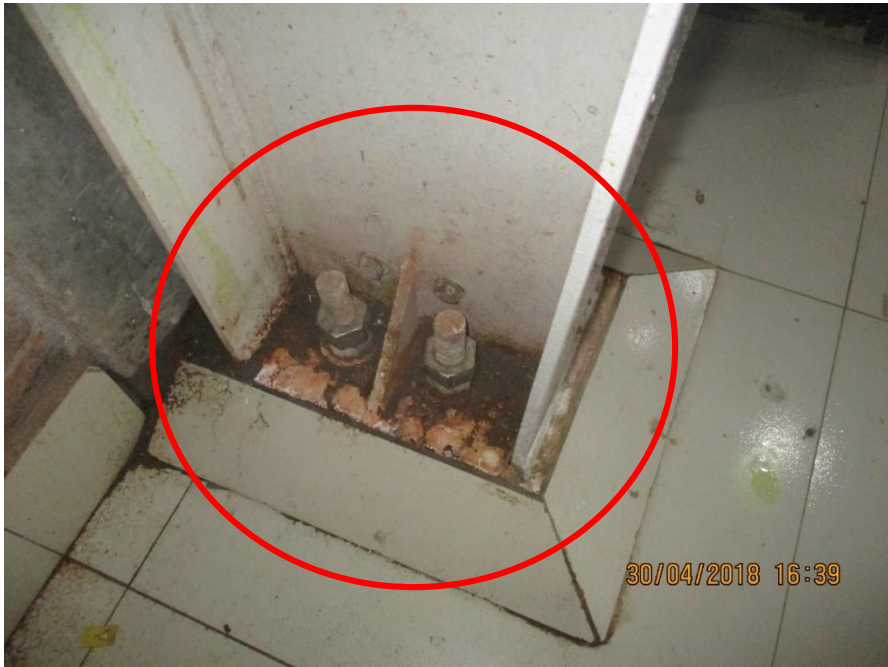
Corrosion observed at Steel column at ground floor
