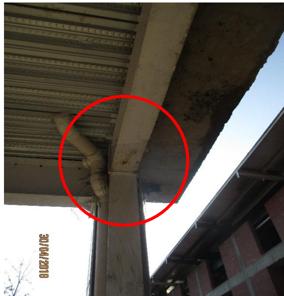
Corrosion was observed on steel columns. Factory is required to identify the locations and take proper remedial measures.
