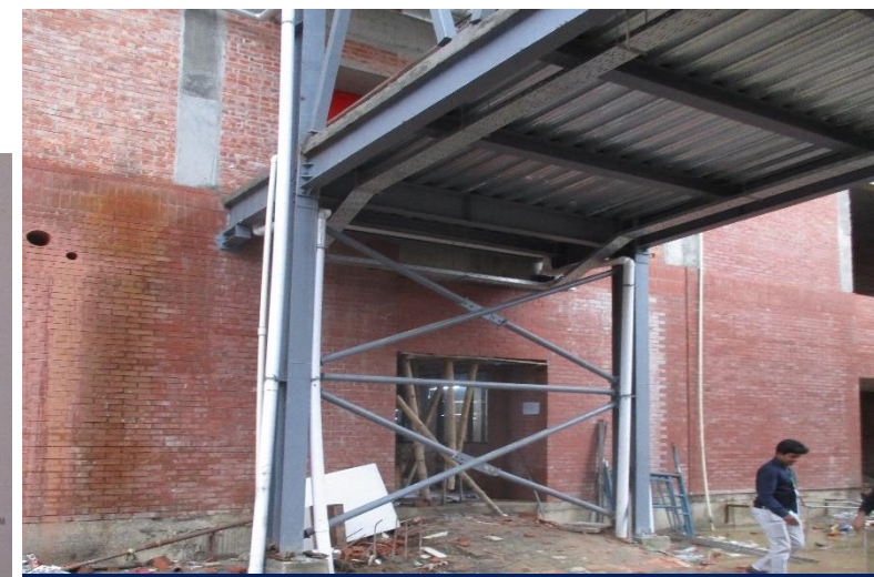
Provided bracing is blocking exit point. Building engineer is required to review design and replace bracing system.
