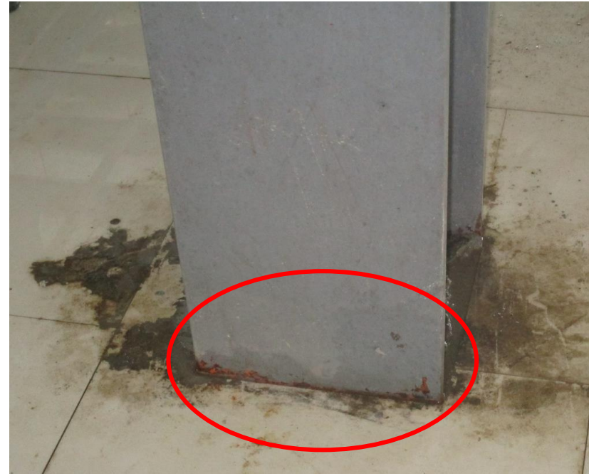
Corrosion was observed at joint of deck slab and steel column in 1 st floor
