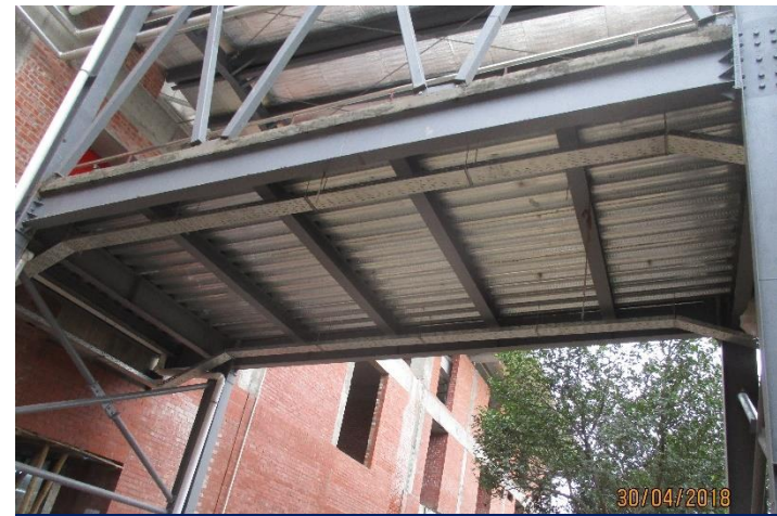
Frame not installed as per drawing
