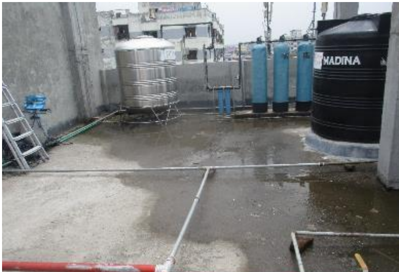
Standing water on roof
