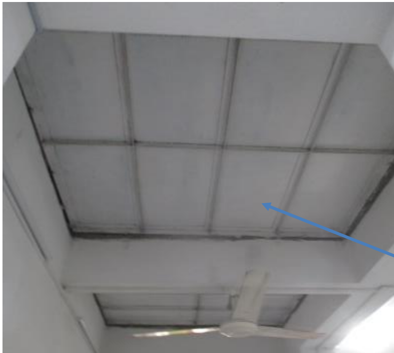
Slab opening covered by steel sheet
