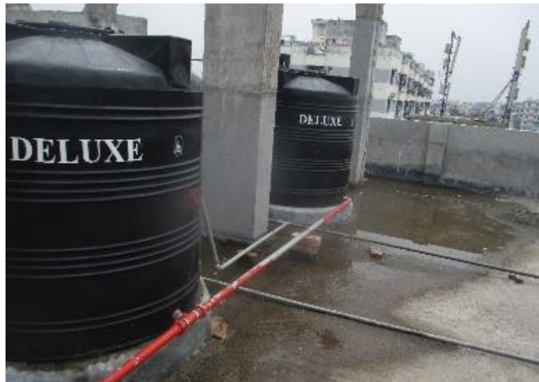
Standing water on roof
